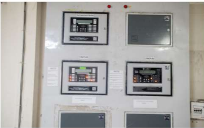
Fire Control Panel
