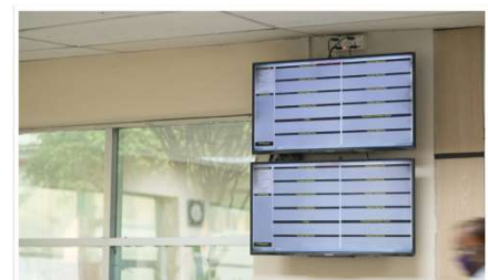
Central Access Management Monitoring System
