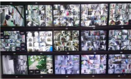
CCTV Camera Control Room
