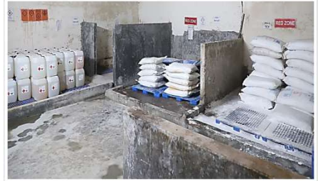
Chemical Store(Red Zone)
