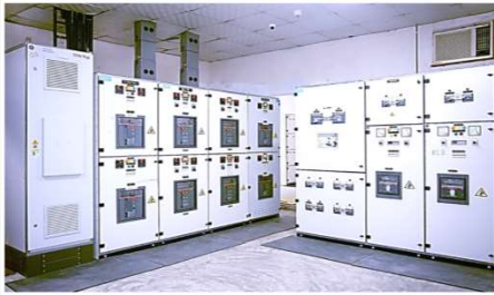
Generator Control Panel
