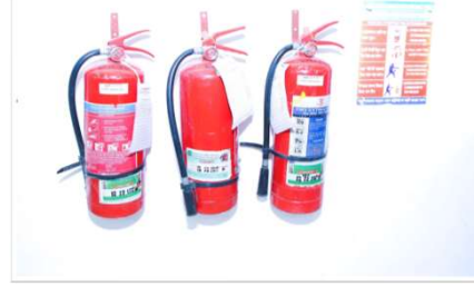
Fire and Safety Equipment
